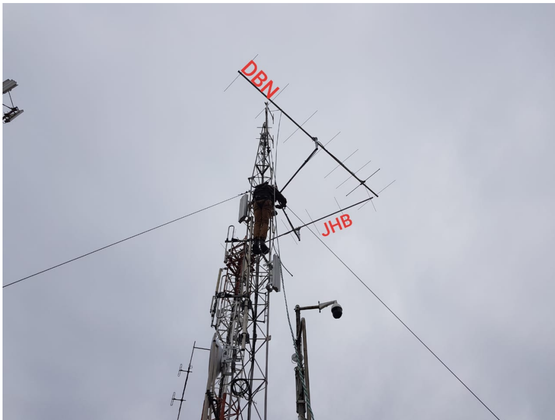
The current analogue beacon in Bethlehem (FreeState Province) The beacon will be replaced with the next generation beacon
